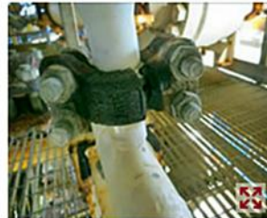
Cracking caused by poor heat treatment during manufacturing process
